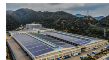
Solar panels in the sorting hub
