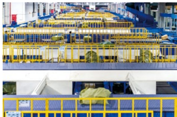
Automated sorting equipment for bulky parcels
